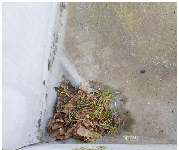
Figure 51- organic debris is blocking some drains
