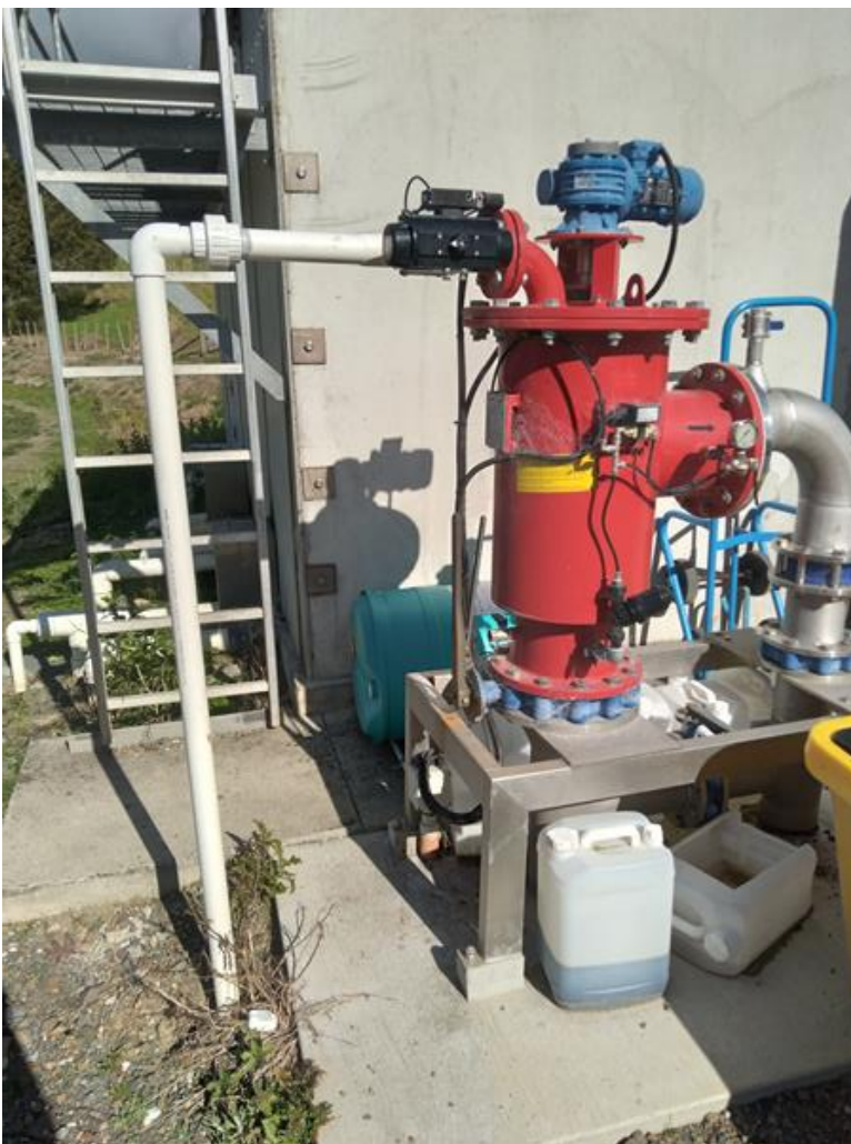
Amiad prefilter for the Maungaturoto WWTP
